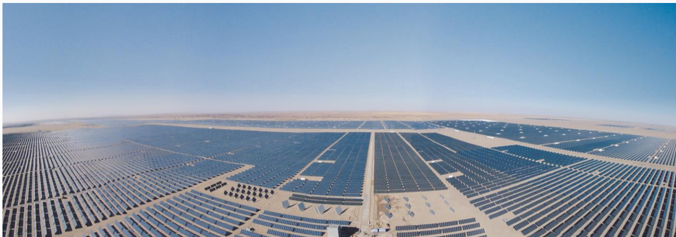
Qianhua Smart PV Plant, 100MW, Tuoketuo, Inner Mongolia, China
